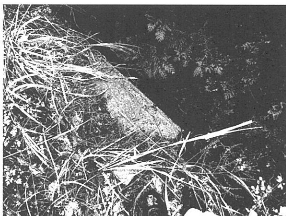
図-2 滑動した擁壁 Fig.2 the retaining wall sliding in the earthquake
